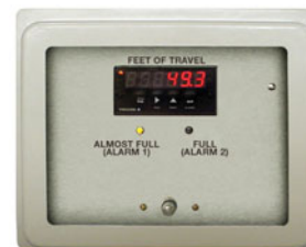
Digital Meter in Outdoor Enclosure with Alarm Lights ▲
