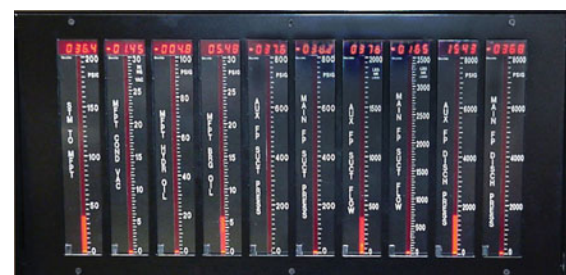
Bargraph Draft Gauges in Rack Panel ▲
